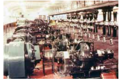
The underground pumping station, located 2.7 miles west of the Red Hill site, has 11 pumps. Photo courtesy of 14th Naval District, Pearl Harbor.
