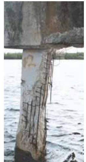
Examples of structurally deficient bridges damaged by corrosion.
