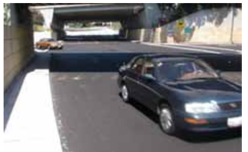
The Castillo Street Underpass is shown 'before' and 'after' an electro-osmotic pulse (EOP) system has been installed. Photo courtesy of Army Corps of Engineers.
