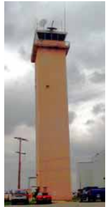
Applying surface-tolerant coatings to structures like this Campbell Army Airfield flight tower requires very little substrate preparation.
