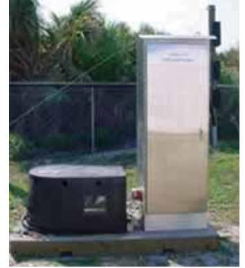
A dehumidification cabinet placed on Daytona Beach is one of several Air Force test samples in an ongoing study of dehumidification methods. Photo courtesy of Air Force Corrosion Office.
