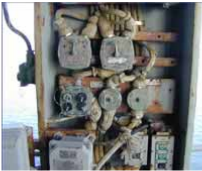
Corroded brass electrical boxes are a costly and time-consuming maintenance problem on Navy vessels. Photo courtesy of NAVSEA.
