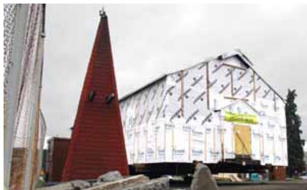
With its steeple dismantled and sitting on the ground, the chapel is hoisted up on wheels and is ready for its journey. Photo by Kayla Overton, USACE Seattle District.
