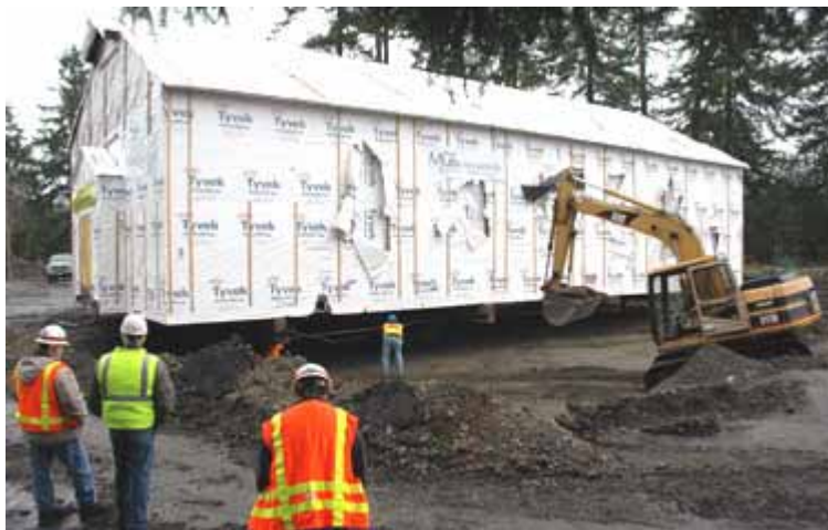
Rich Littooy, Barry Poirrer, and Elizabeth Chien, all of the Corps of Engineers' Seattle District, observe as the chapel is placed into its new location. Photo by Kayla Overton, USACE Seattle District.
