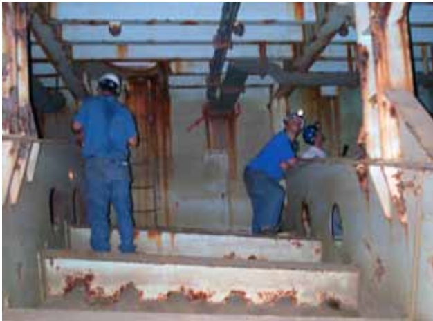
The Naval Research Lab has developed a table-top, computer-based system to improve upon the Navy's physical method of assessing ballast tank coatings. From left, Navy corrosion experts Rich Hays, Ted Lemieux, and Bill Groeninger inspect the tank interior of an LSD 41 amphibious combatant ship in 2002. Photo courtesy of Paul Slebodnick, Naval Research Lab.
