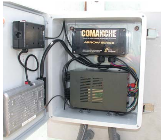
FIGURE 1b- Typical RMU installed on water storage tanks at Army Installation #1
