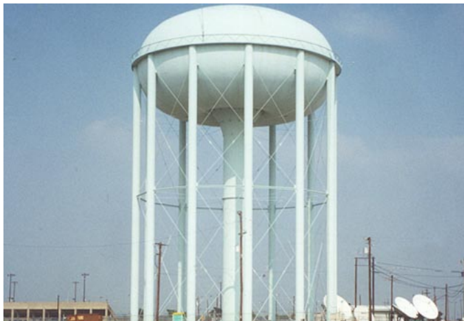
FIGURE. 1a- Elevated 2 MMG potable water storage tank at Army Installation #1
