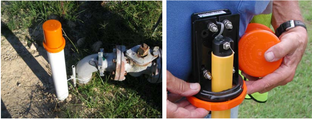
FIGURE 4- Left: Typical Pipe Protection Remote Monitoring Units Installed to Interrogate the Pipeline and Transmit System Corrosion Control Effectiveness Data. Right: Remote Monitor Unit with Cap Removed Showing Terminal Connection Points
